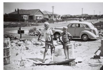
Figure 30 John and Tony Berens helping with house building activities, St James, Perth c1951. Courtesy: Berens Family.
